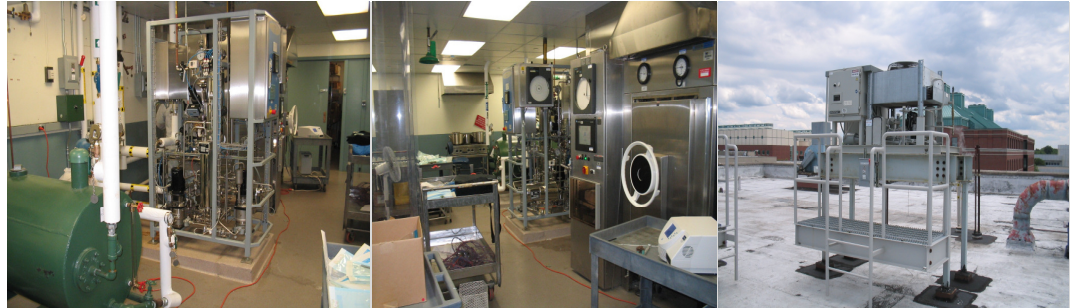
Clean Steam Generator
